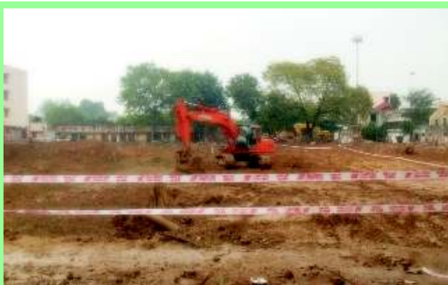
Construction of Emergency Block under Redevelopment Scheme of Safdarjung Hospital, New Delhi
