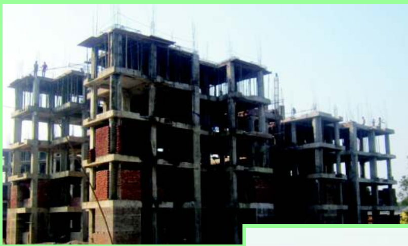
The Up-gradation work at Lokopriya Gopinath Bordoloi Regional Institute of Mental Health (LGBRIMH), Tezpur, Assam
