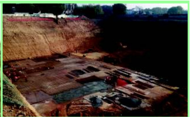
Construction of Super Specialty Block under the Redevelopment Scheme of Safdarjung Hospital, New Delhi
