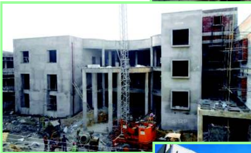
Construction of Nursing College consisting of multi-purpose Hall, Laboratory, Library Facility & Common Room etc. at Govt Medical College, Patiala
