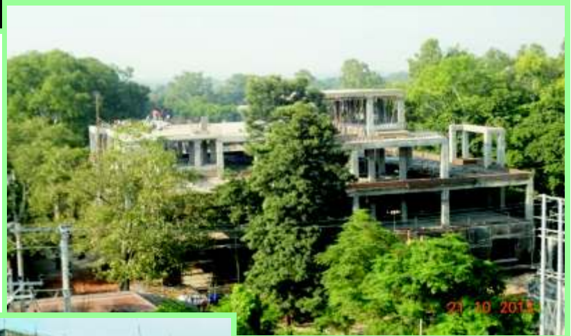
Construction of GPL Standard Invivo Laboratory at Indian Institute of Integrative Medicine (IIM), Jammu
