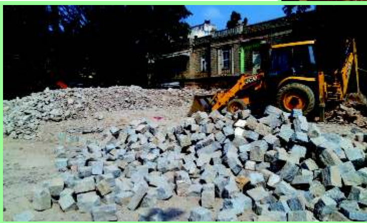
Construction of 42 bed Metro Block ( High Risk Pregnancy Ward ) in the Campus of Vani Vilas Hospital, Bengaluru
